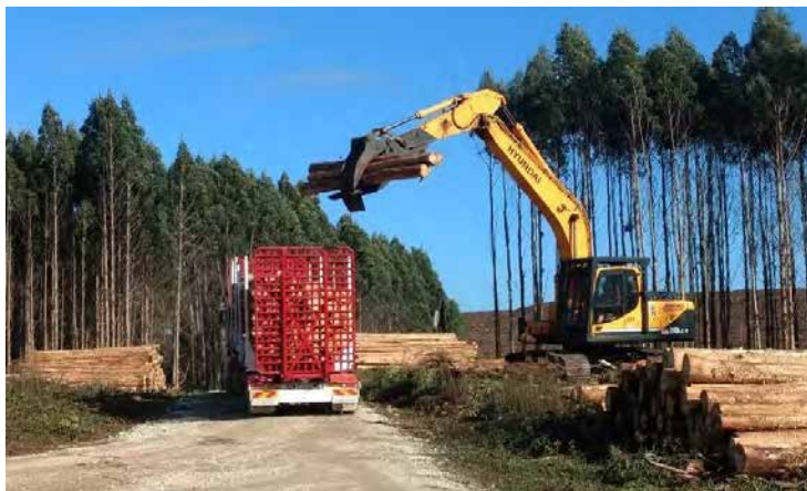
Loading plantation logs during a Forico operation. This year saw a drop in new plantations on previously cleared land (62 hectares this year and 173 last year) and in new plantations on cleared native forest sites (48 hectares this year and 72 hectares last year).
